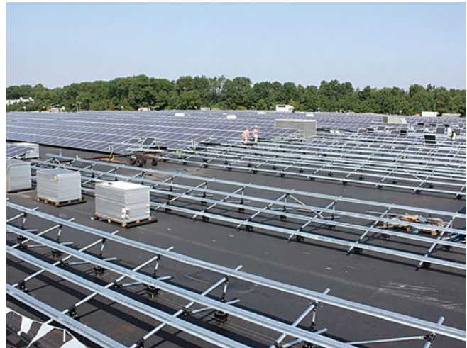
For the Parsippany facility, Silverback engineered a racking structure with 16 degrees of tilt and plenty of working clearance beneath to allow for maintenance on the 18-year-old roof membrane.
